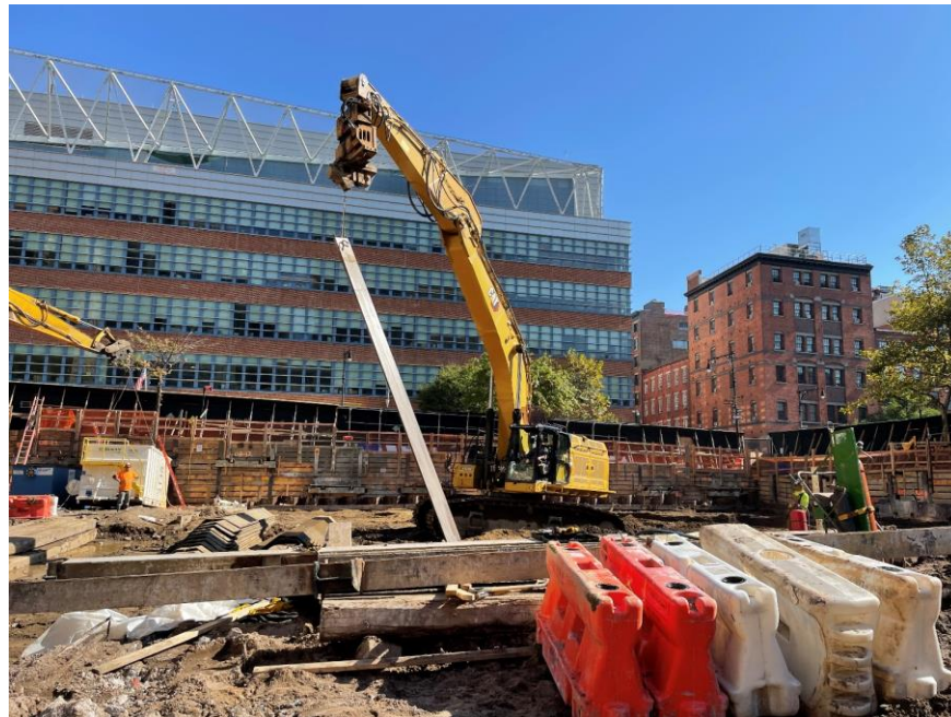
Photo 1: CCJV removing previously installed steel sheet piles in the southeastern part of the site (facing east)
