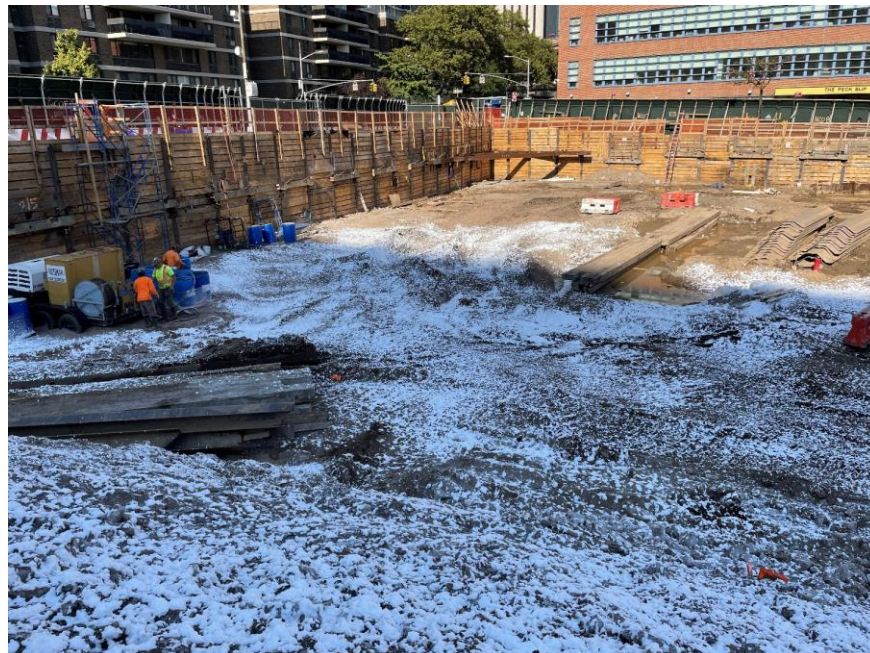
Photo 2: Exposed soil/fill covered in Atmos® AC-645 dust/vapor suppressing foam for the temporary overnight cover (facing northeast)
