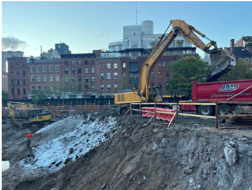
Photo 1: CCJV applying Atmos® AC-645 dust/vapor suppressing foam during excavation and live-loading of non-hazardous soil/fill (facing south)
