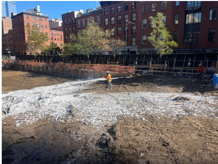
Photo 2: CCJV applying Atmos® AC-645 dust/vapor suppressing foam to exposed soil/fill for the temporary overnight cover (facing southwest)
