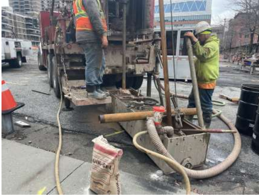
Photo 1: Craig preparing to advance a geotechnical boring in the southwestern part of the site (facing east)
