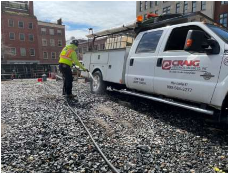
Photo 2: ECD washing a vehicle on the tracking pad prior to exiting the site (facing southwest)
