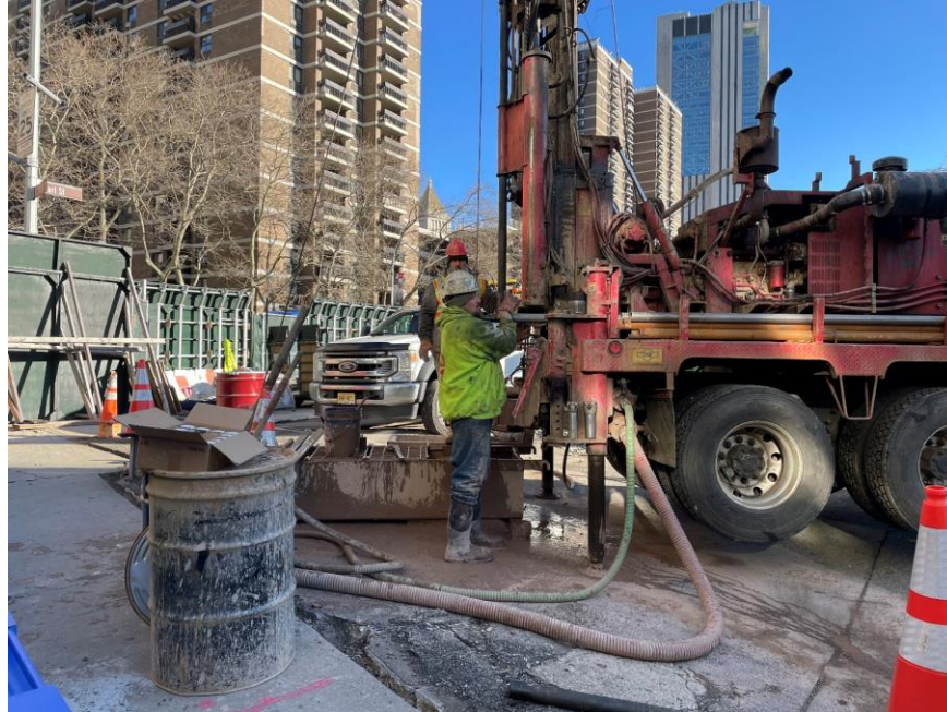
Photo 1: Craig advancing a geotechnical boring in the northwestern part of the site (facing northeast)
