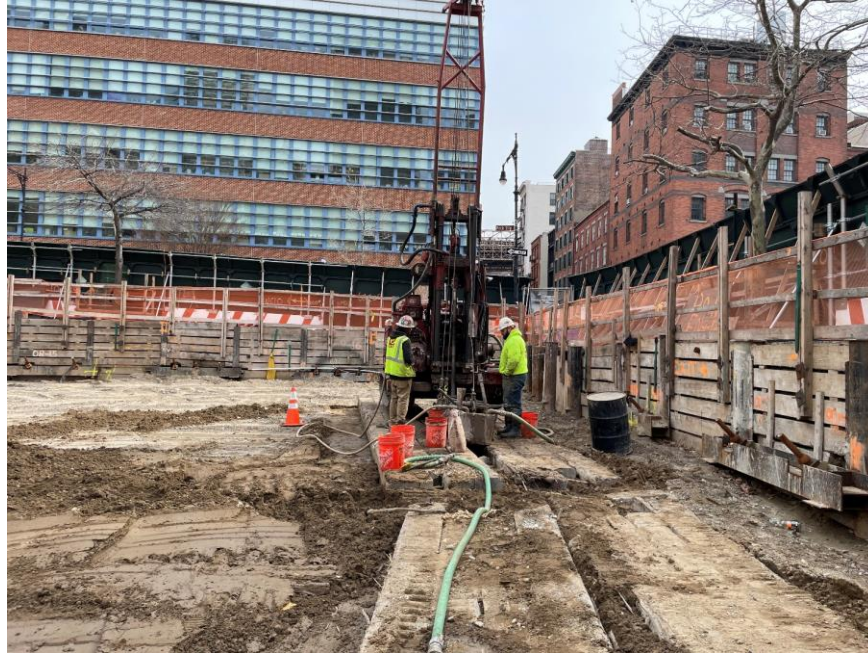
Photo 1: Craig advancing a geotechnical boring in the southeastern part of the site (facing east)
