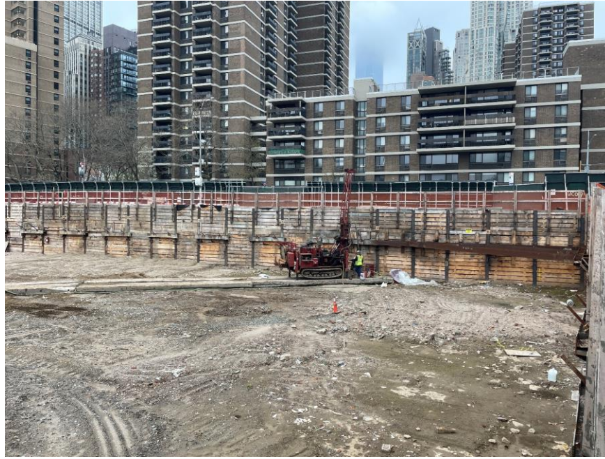
Photo 1: Craig advancing a geotechnical soil boring in the northeastern part of the site (facing north)
