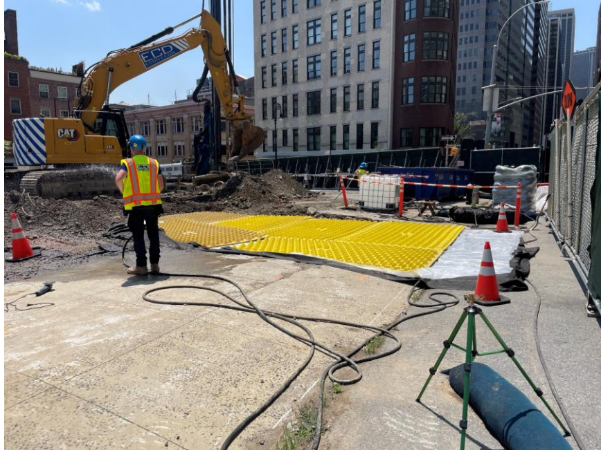
Photo 1: Stabilized construction entrance in the northwestern part of the site (facing west)
