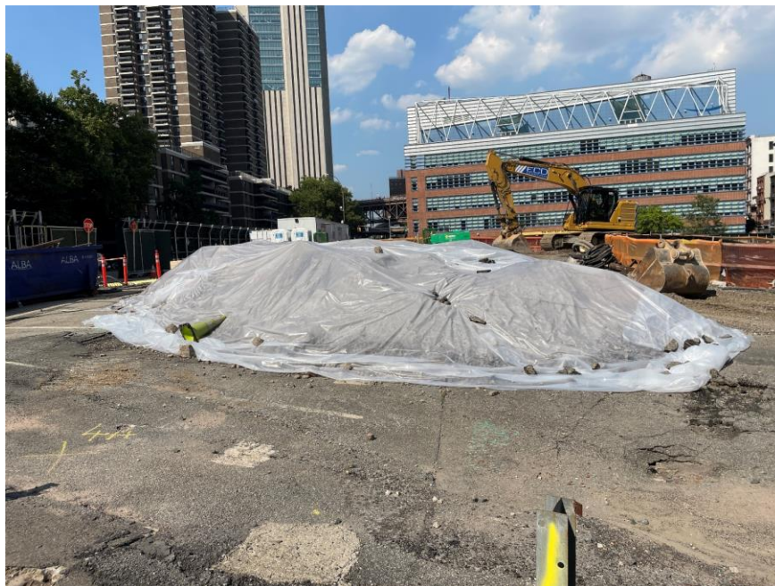
Photo 2: Soil/fill stockpile on and covered with polyethylene sheeting in the northwestern part of the site (facing northeast)
