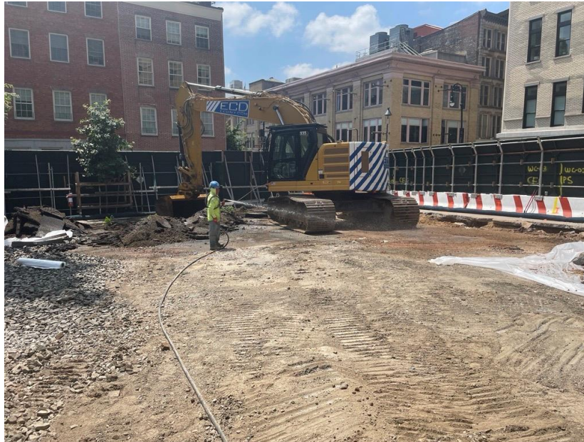
Photo 1: ECD excavating soil/fill in the southwestern part of the site (facing southwest)
