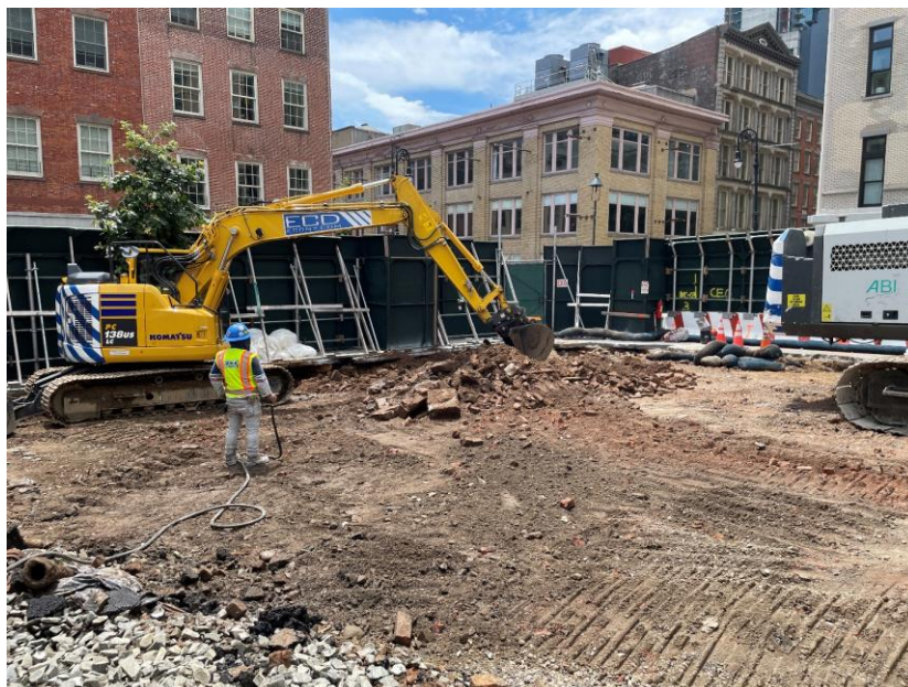
Photo 2: ECD excavating soil/fill in the southwestern part of the site (facing southwest)
