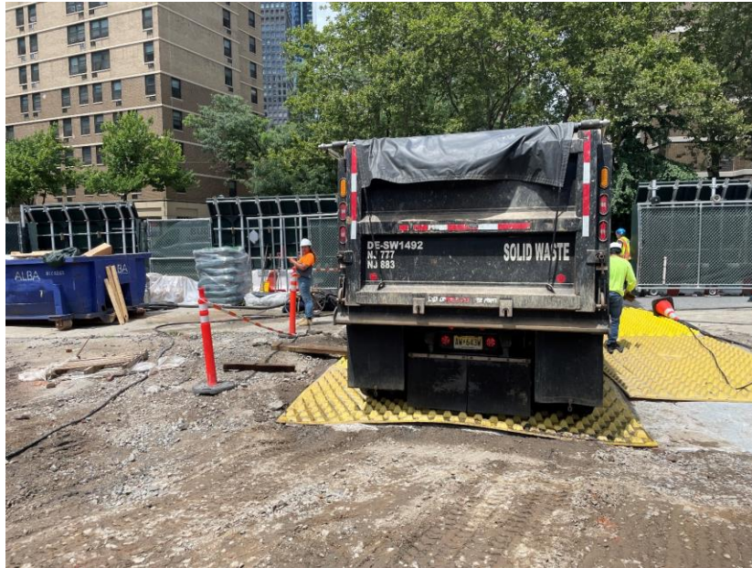
Photo 1: ECD washing a tri-axle truck prior to exiting the site (facing north)
