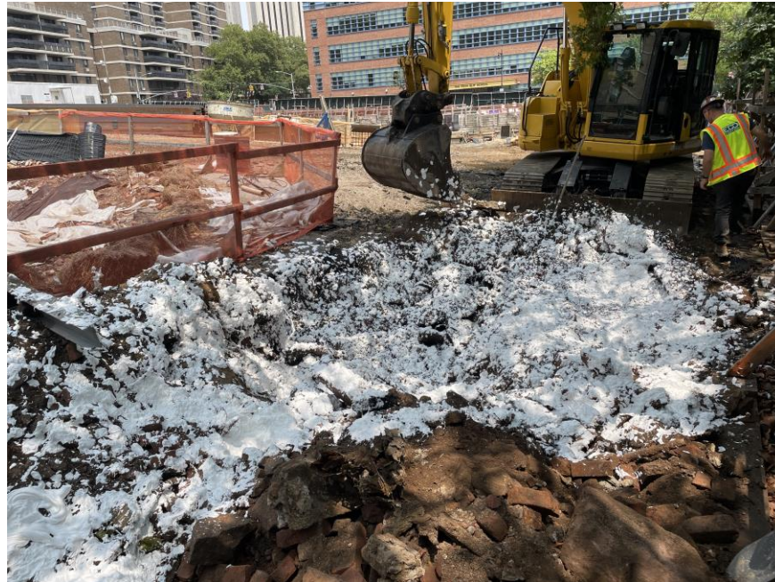
Photo 1: ECD actively applying Atmos® AC-645 dust/vapor suppressing foam to soil/fill during excavation in the southern part of the site (facing northeast)
