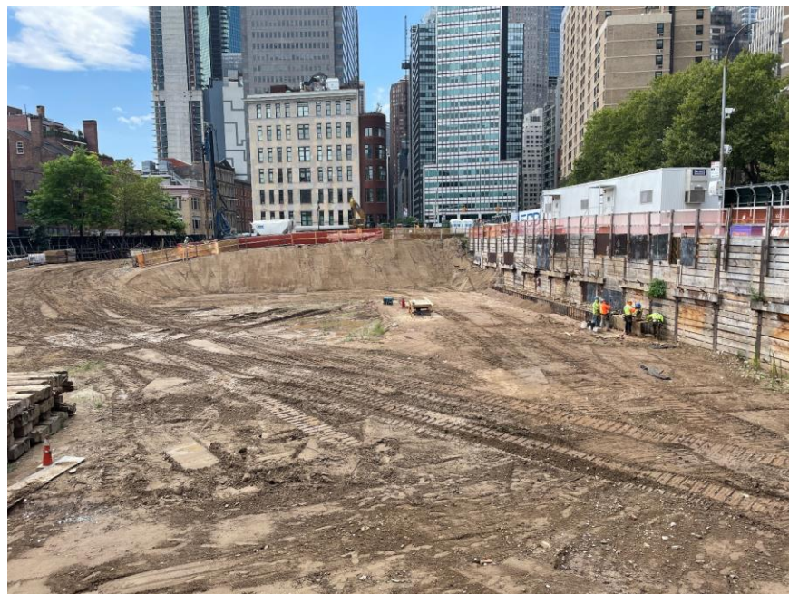
Photo 2: ECD constructing wooden formwork in preparation for concrete guide wall installation in the northern part of the site (facing west)
