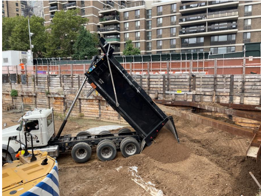
Photo 1: ECD importing general fill atop polyethylene sheeting in the northeastern corner of the site (facing northwest)
