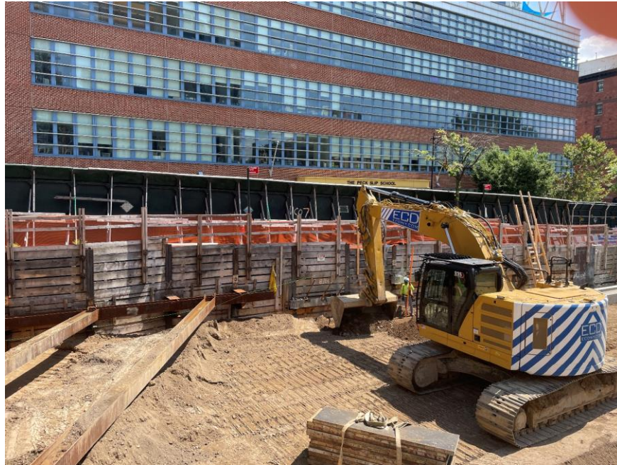
Photo 1: ECD grading imported general fill in the northeastern part of the site (facing east)
