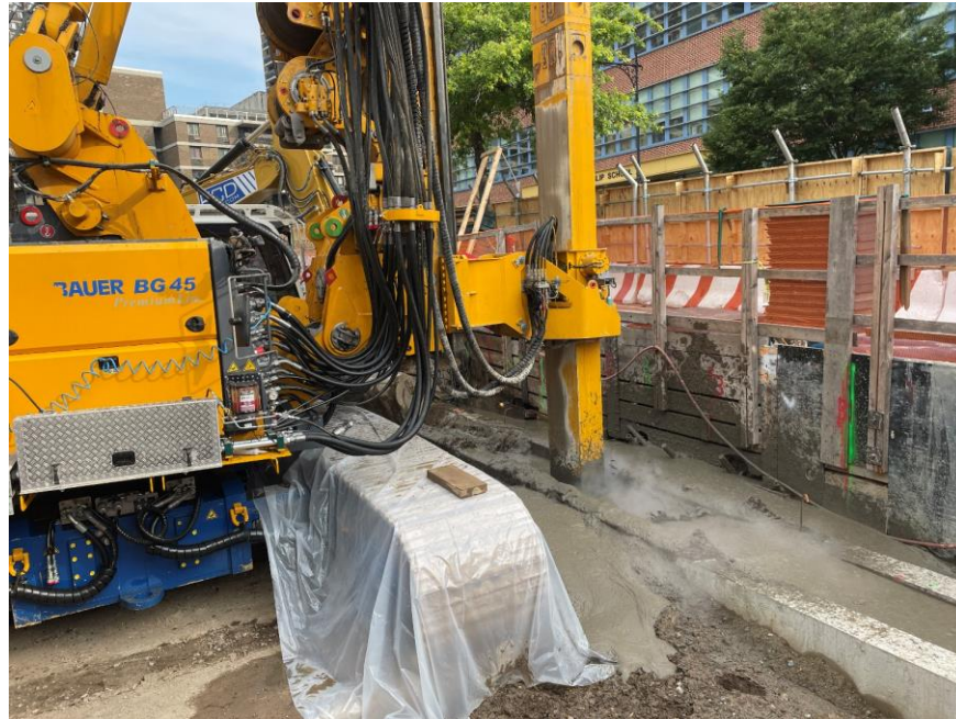
Photo 1: ECD installing a soil mix column in the eastern part of the site (facing northeast)
