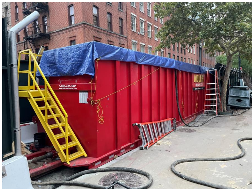
Photo 2: Dewatering tank staged in the southeast part of the site (facing southwest)
