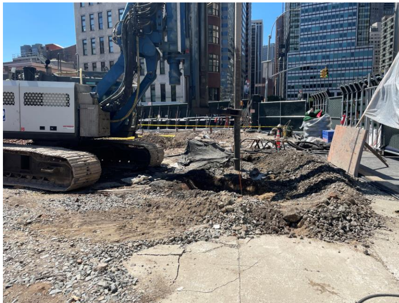
Photo 2: ECD installing a soldier pile in the northern part of the site (facing west)
