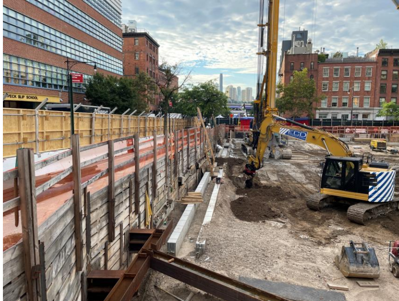
Photo 1: ECD excavating soil/fill in the eastern part of the site (facing south)
