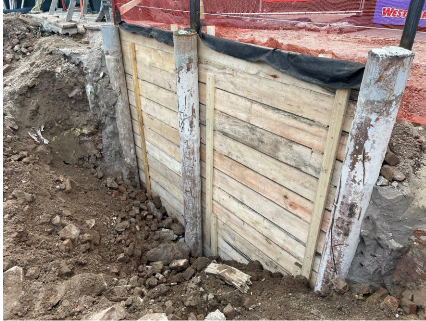
Photo 1: Timber lagging installed along the northern perimeter of the site (facing northwest)
