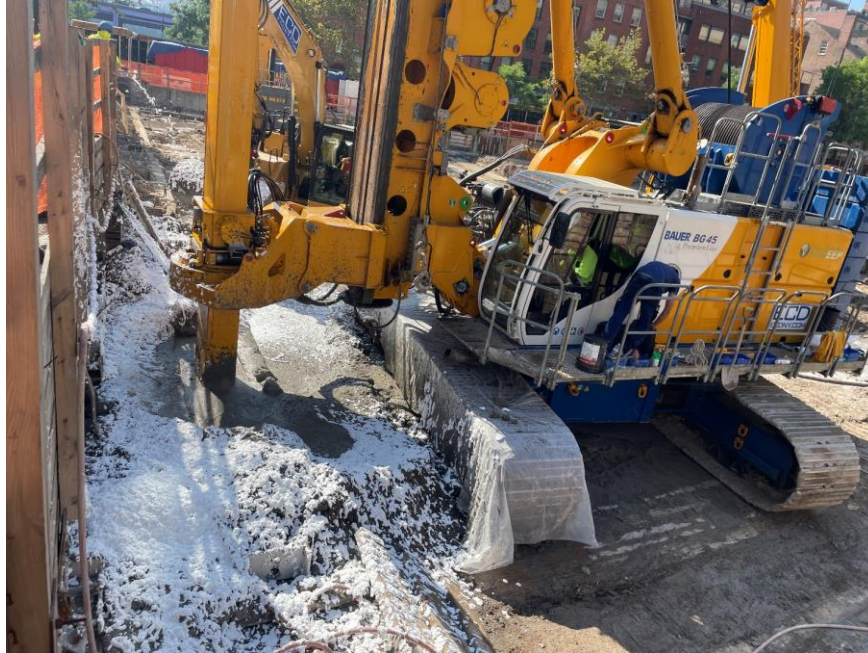
Photo 1: Atmos® AC-645 odor/vapor suppressing foam applied to soil/fill during soil mix column installation in the eastern part of the site (facing south)
