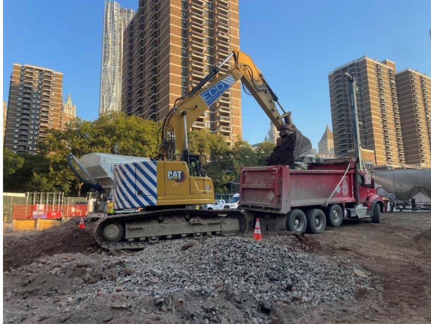
Photo 1: ECD loading a dump truck with soil/fill from the western part of the site for off-site disposal (facing northeast)
