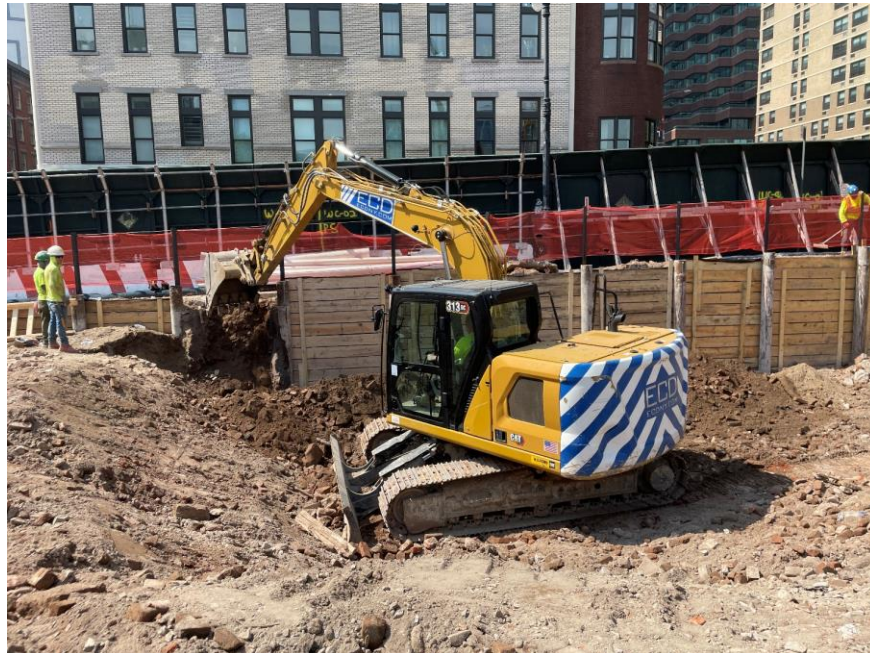
Photo 2: ECD excavating soil/fill in the western part of the site (facing west)
