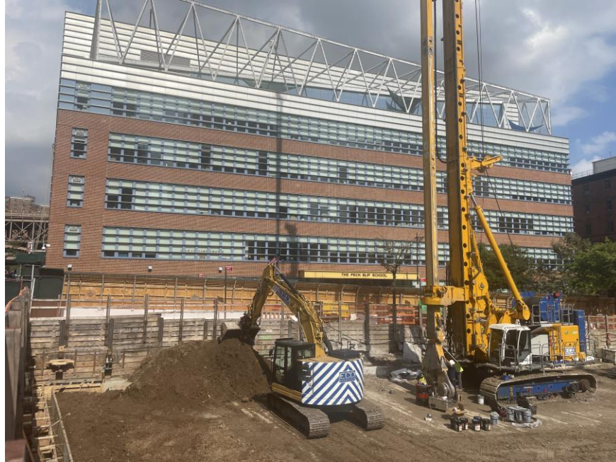
Photo 1: ECD excavating previously imported fill in the northeast part of the site (facing east)
