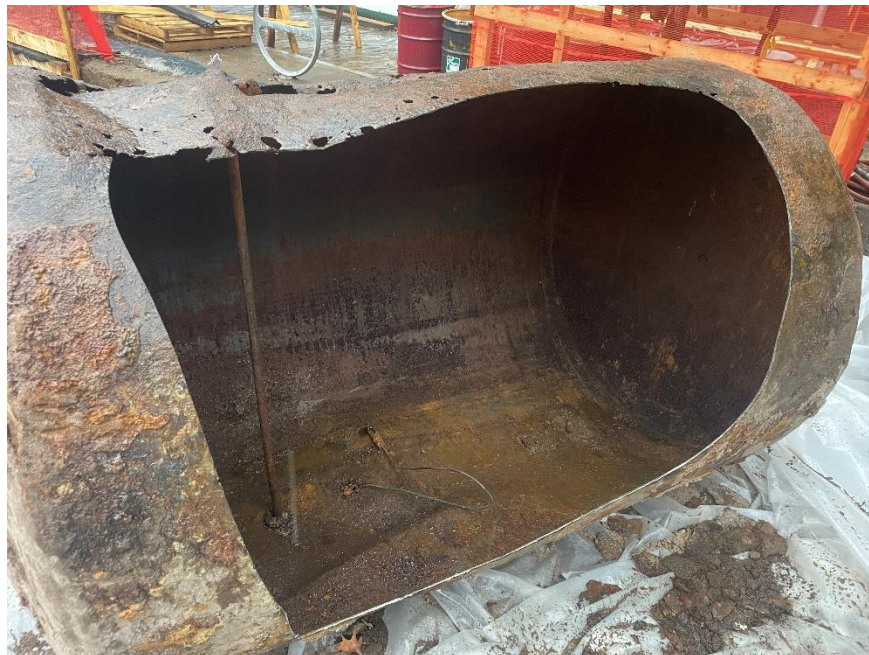
Photo 2: Decommissioned UST in the southern part of the site prior to off-site disposal (facing southeast)
