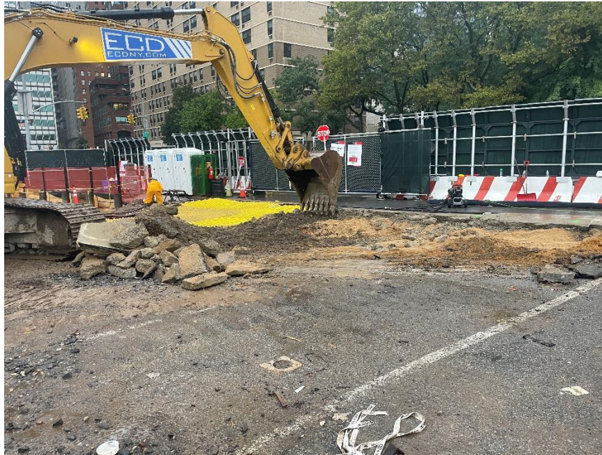
Photo 1: ECD demolishing existing asphalt and concrete in the northern part of the site (facing northwest)
