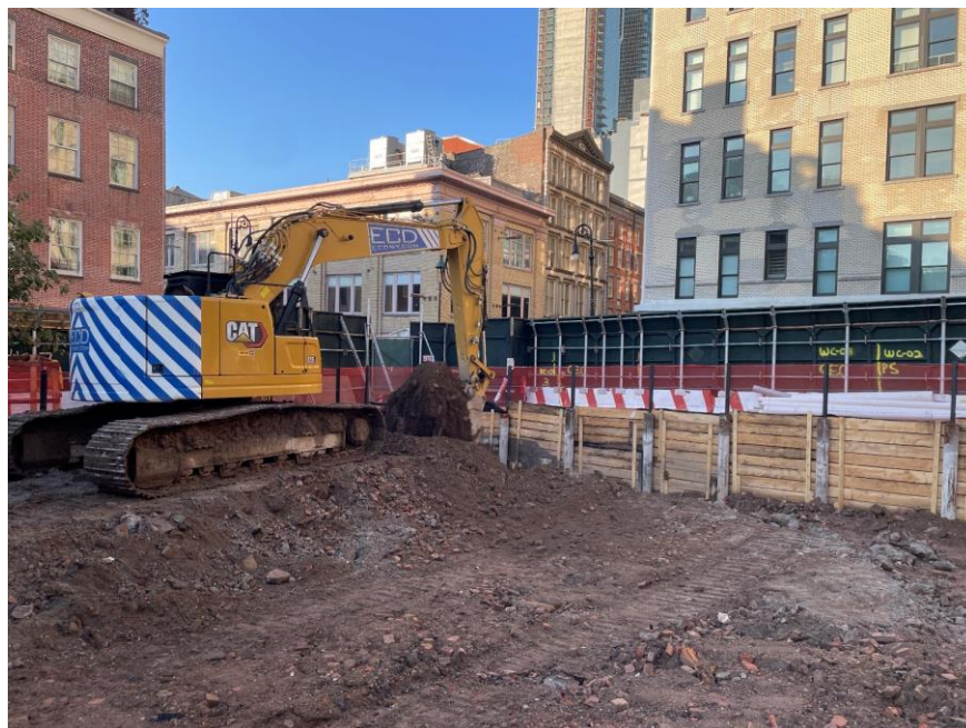
Photo 2: ECD excavating soil/fill in the western part of the site (facing southwest)
