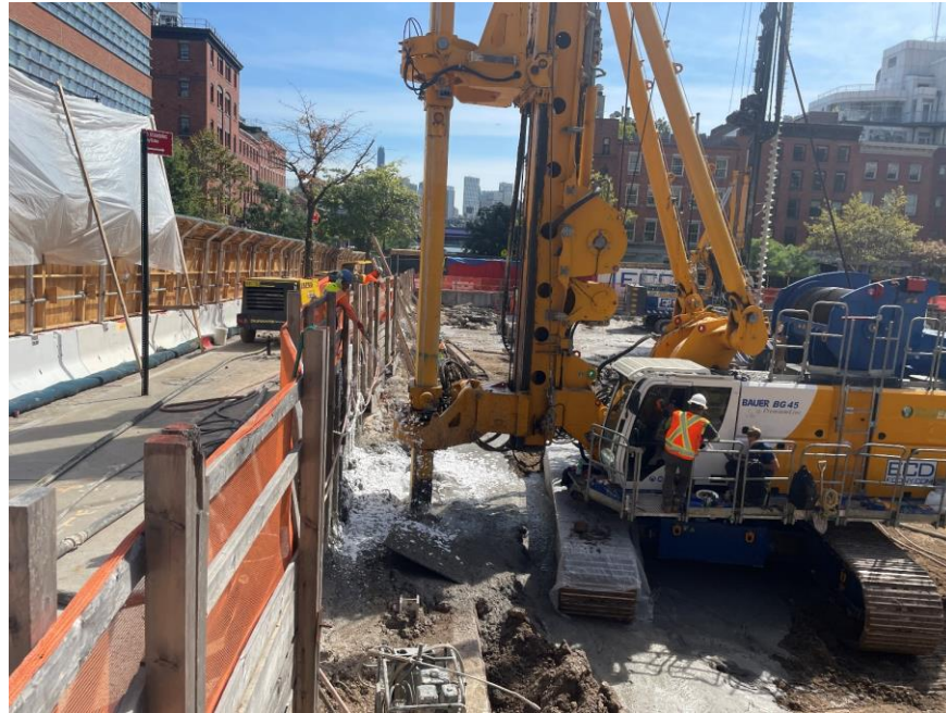
Photo 1: Atmos® AC-645 odor/vapor suppressing foam applied during soil mix column installation in the eastern part of the site (facing south)
