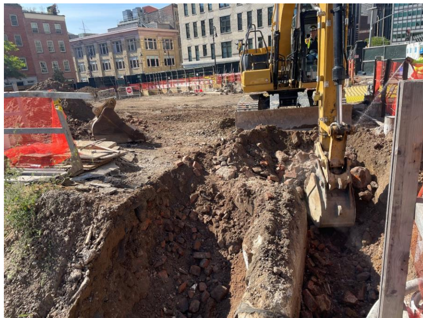
Photo 2: Mercon-X® mercury vapor suppressant applied during excavation in the northern part of the site (facing west)
