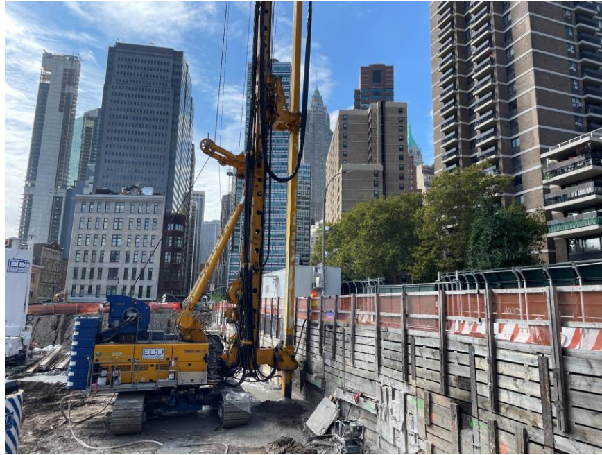
Photo 1: ECD installing a soil mix column in the northeast part of the site (facing west)
