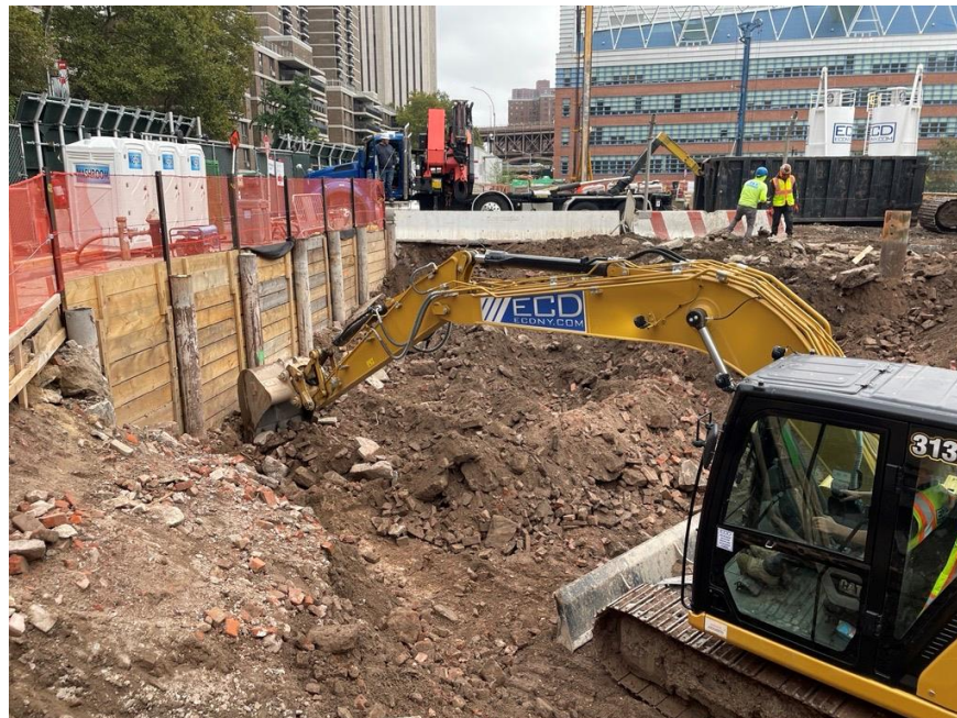
Photo 2: ECD excavating soil/fill in the northwest part of the site (facing east)
