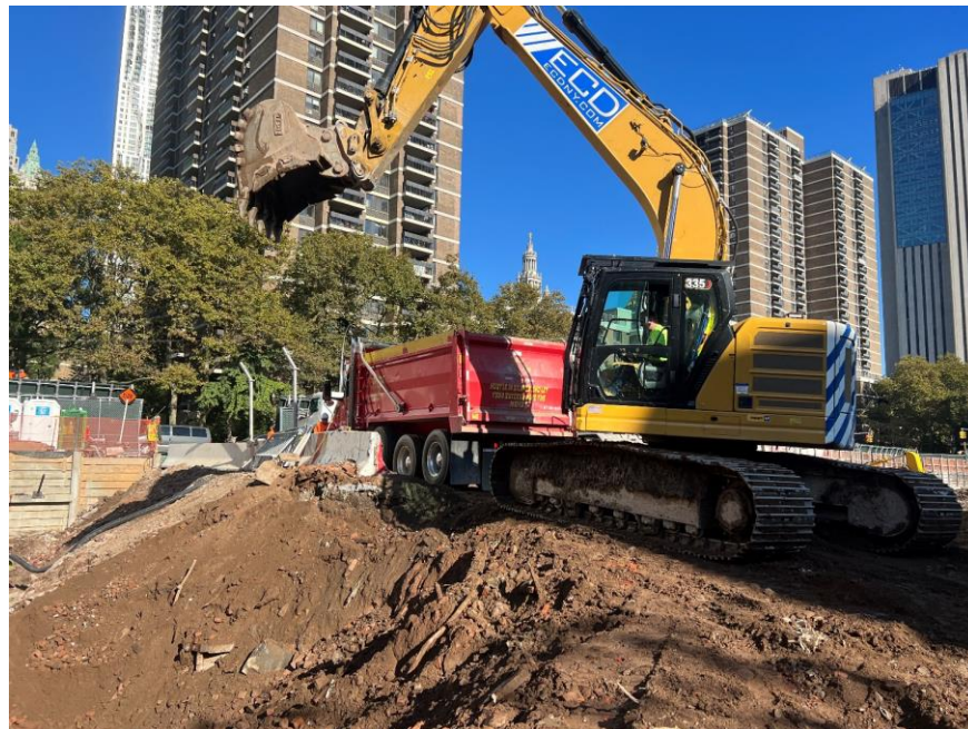
Photo 2: ECD loading a truck with C&D debris for off-site disposal (facing north)
