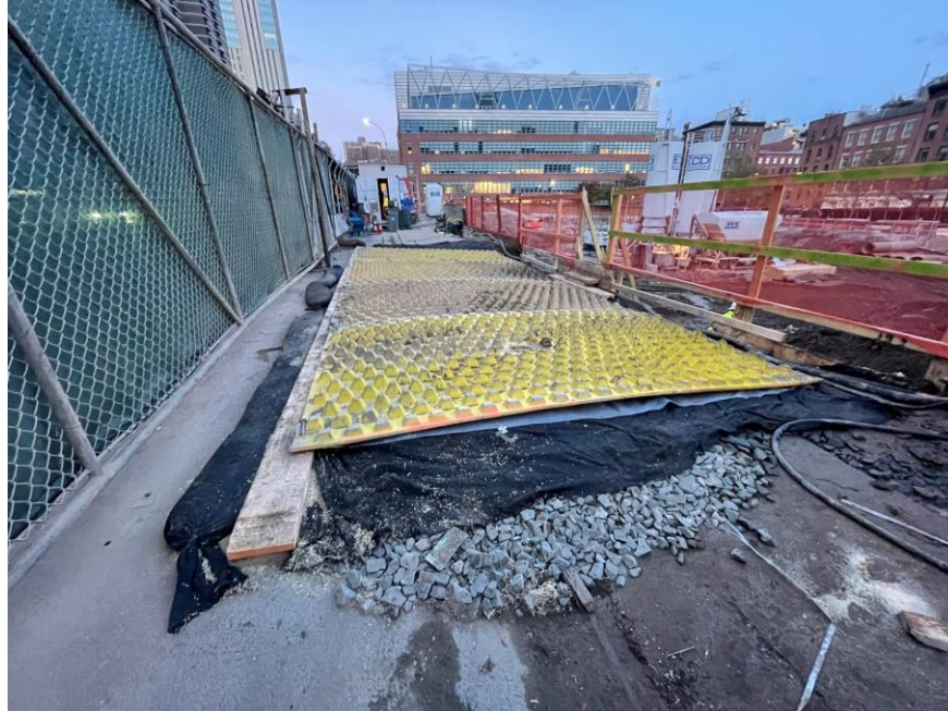
Photo 1: Stabilized construction entrance installed in the northwest part of the site (facing east)
