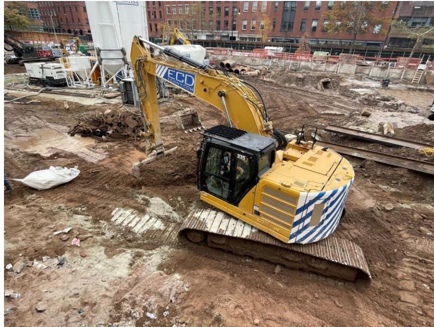
Photo 1: ECD excavating soil/fill in the north-central part of the site (facing south)
