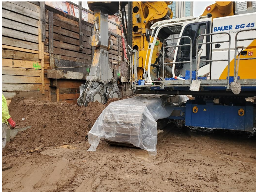
Photo 2: ECD installing a soil mix column in the southern part of site (facing southwest)
