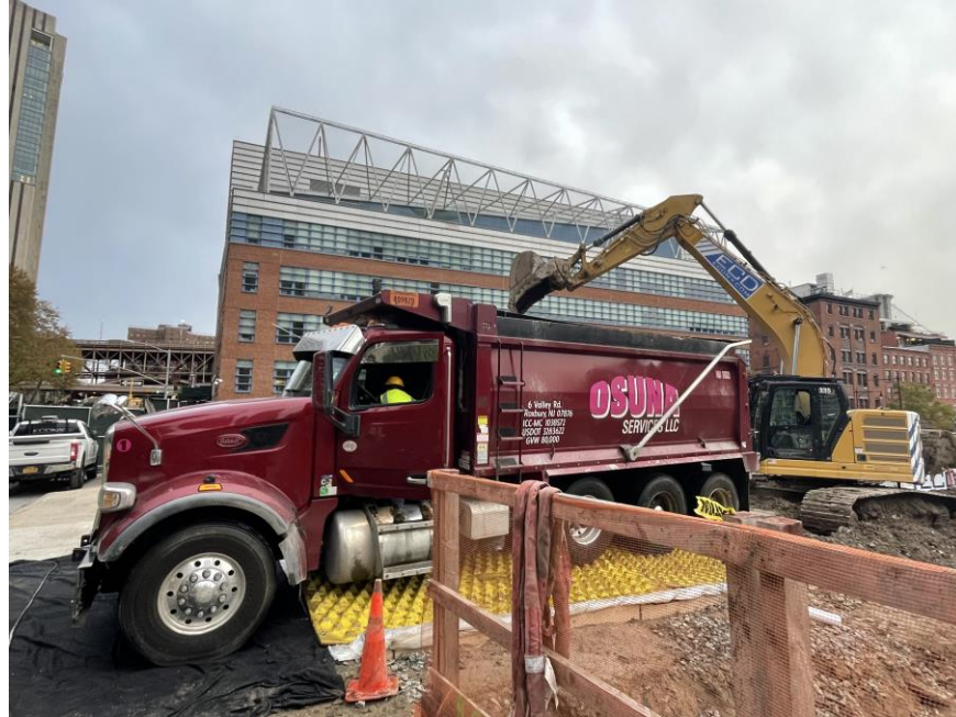
Photo 1: ECD loading a truck with non-hazardous soil/fill for off-site disposal (facing east)
