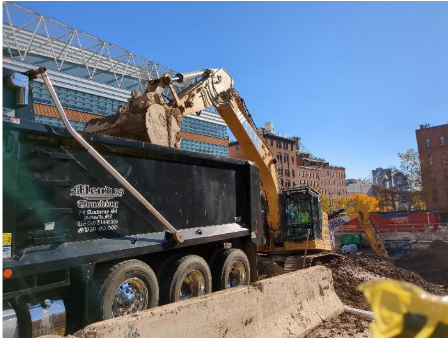
Photo 1: ECD loading a truck with non-hazardous soil/fill for off-site disposal (facing southeast)
