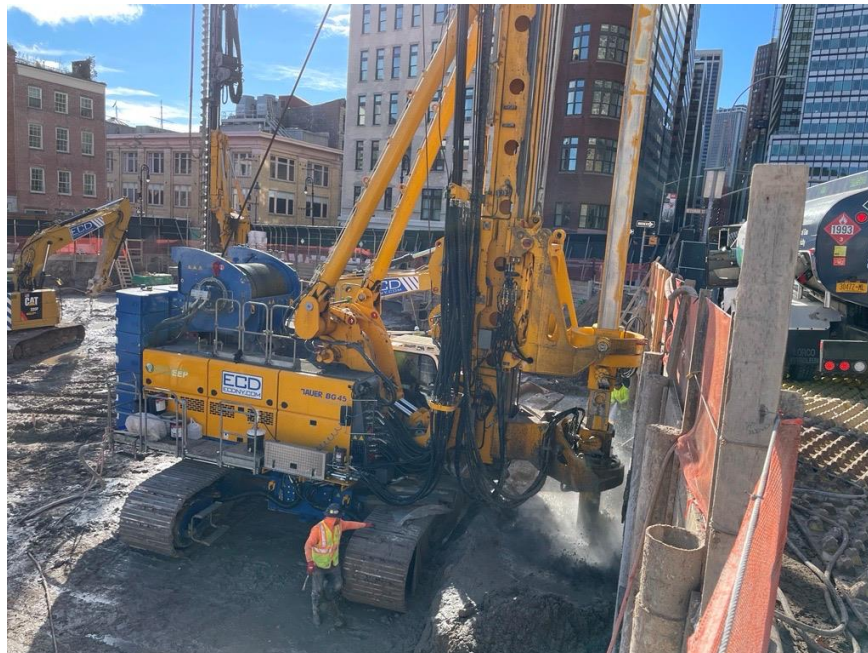
Photo 2: ECD installing a soil mix column in the northern part of site (facing west)
