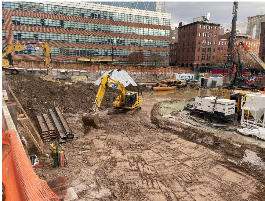
Photo 1: ECD grading soil/fill in the northern part of the site (facing southeast)
