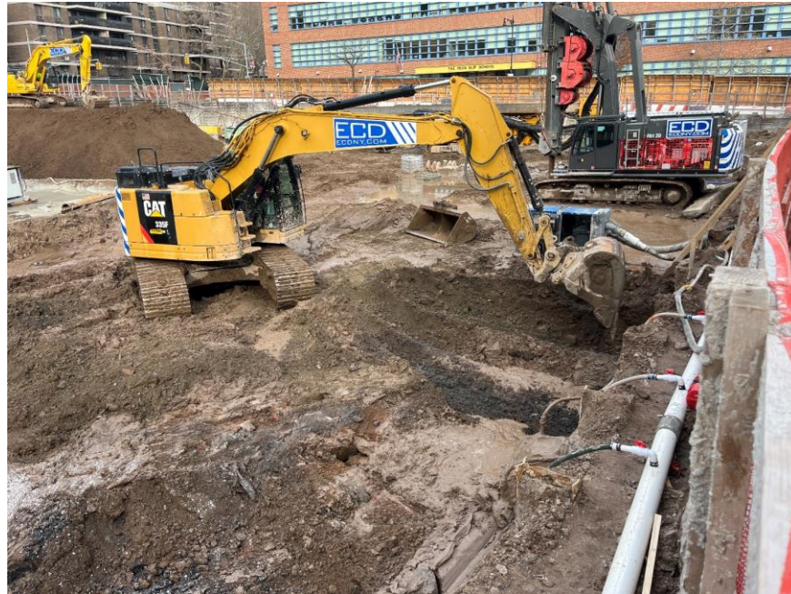
Photo 1: ECD excavating soil/fill in the southern part of the site (facing north)
