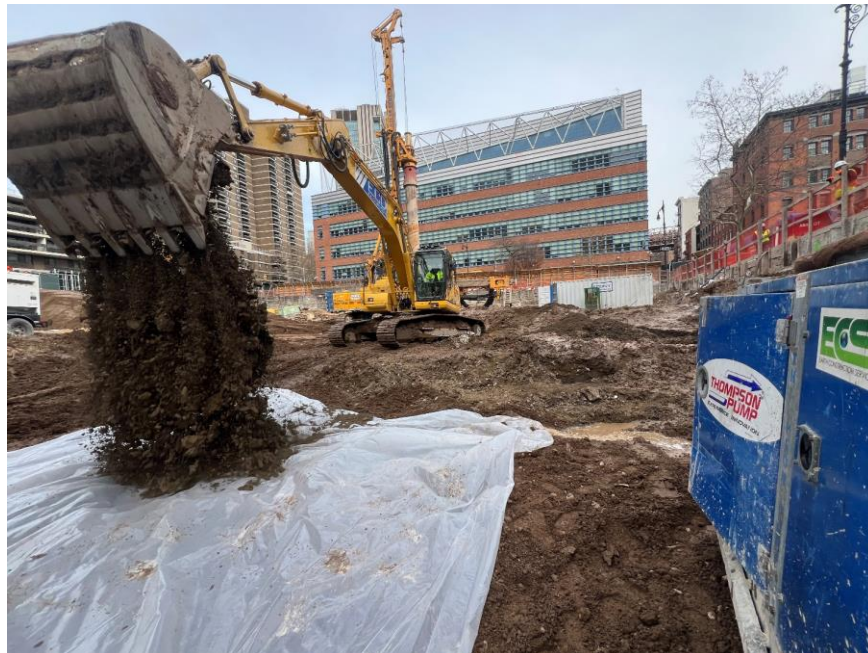
Photo 2: ECD excavating non-hazardous soil/fill in the southern part of the site (facing east)
