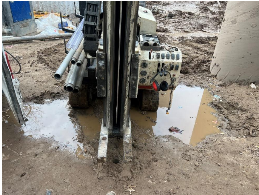
Photo 2: Lakewood installing temporary monitoring well TMW36 in the southeast part of the site (facing west)
