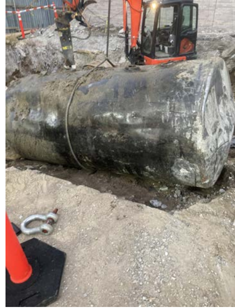
6. Upon completion of removal and cleaning of UST contents, each UST is removed from the ground.
