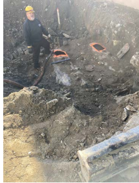
10. Additional USTs located with contents removed.
