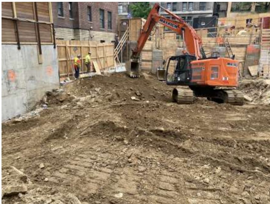
Photo 8: View of Mayrich excavating non-hazardous historical fill and native soil in the northwestern part of the site, facing northwest. Taken on 06/01/2022
