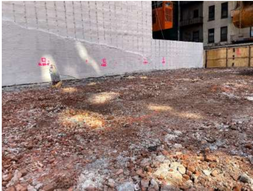
Photo 1: View of site prior to mobilization for excavation activities, facing southeast. Taken on 05/09/2022
