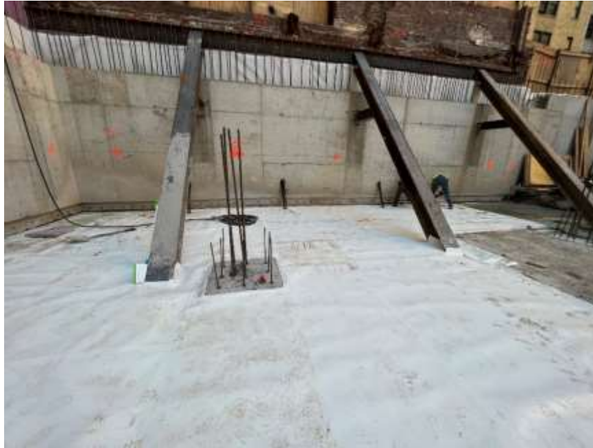
Photo 13: View of waterproofing installed in the southern part of the site, facing south. Taken on 07/27/2022
