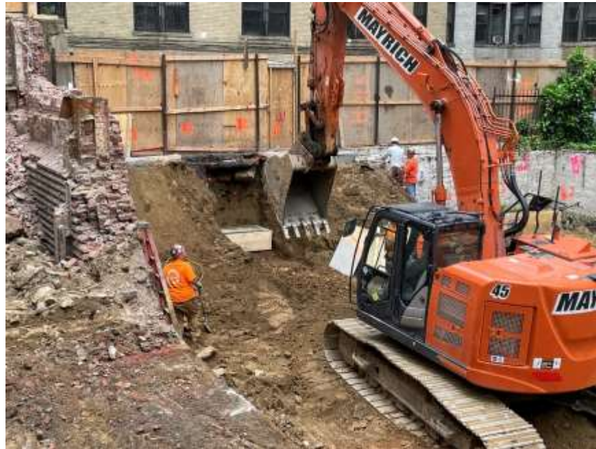
Photo 6: View of Mayrich installing underpinning for the support of excavation (SOE), facing south. Taken on 05/24/2022
