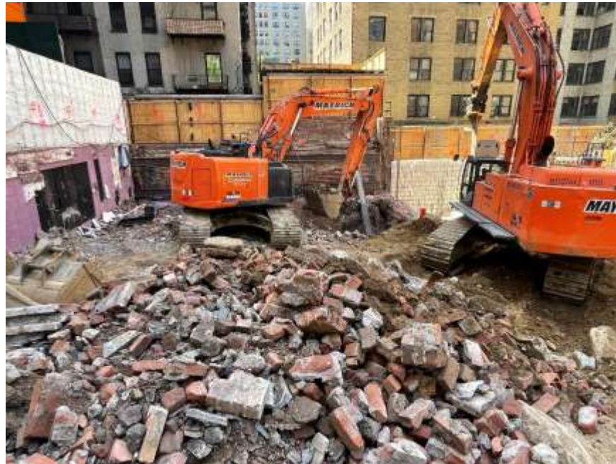
Photo 4: View of Mayrich removing C&D in southeastern part of site, facing south. Taken on 05/15/2022
