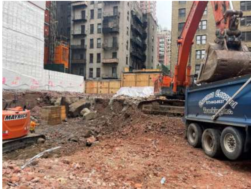
Photo 3: View of Mayrich Construction (Mayrich) loading a truck with construction and demolition (C&D) material for off-site disposal, facing southeast. Taken on 05/13/2022
