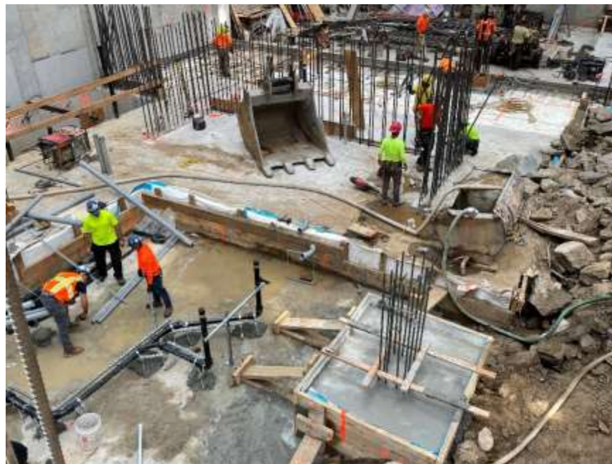
Photo 14: View of the on-site segment of the dewatering system, facing southeast. Taken on 08/08/2022
