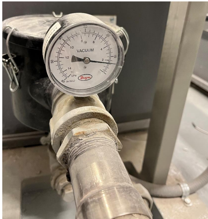
Photo 8, 01/17/2023: Vacuum gauge attached to SMD system blower (facing southwest)
