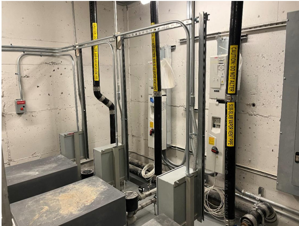
Photo 5, 01/17/2023: View of SMD system effluent vent pipes leading to the building roof (facing northwest)
