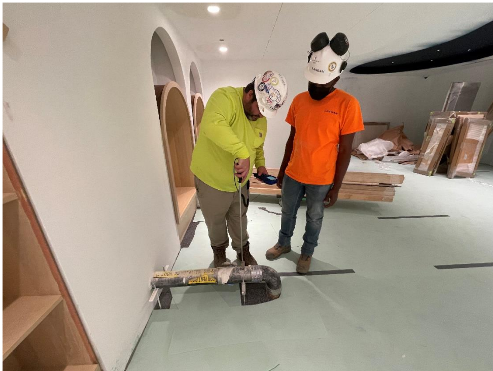
Photo 12, 04/25/2023: Langan using a Velocicalc to measure flow rate within the cellar-level riser pipe connection (facing east)
