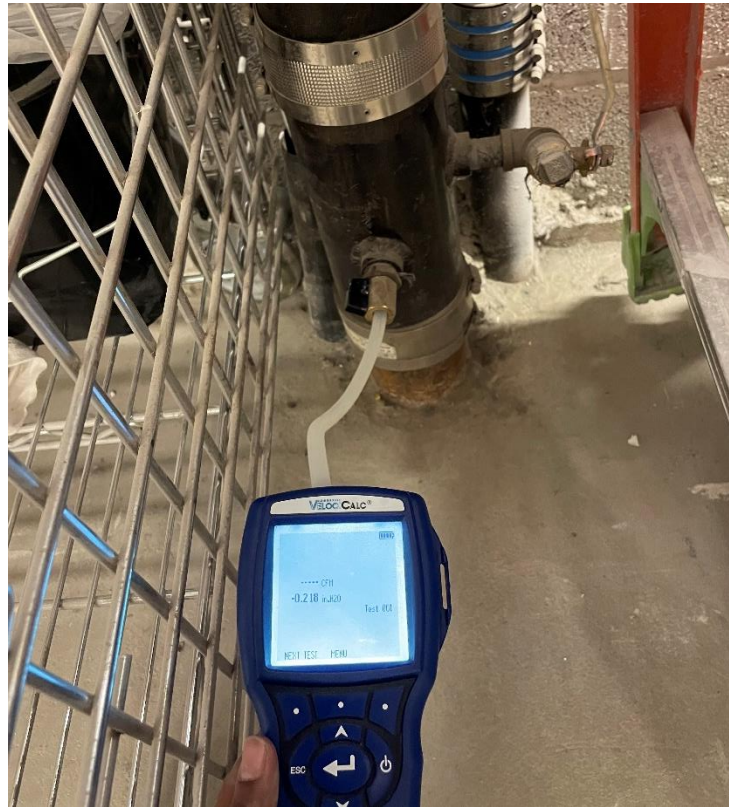
Photo 15, 04/25/2023: View of Langan collecting vacuum readings from the western first floor-level riser pipe connection (facing west)
