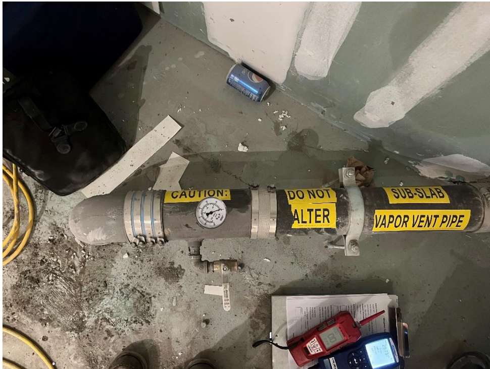
Photo 17, 01/17/2023: View of the completed riser pipe connection exiting the eastern first floor-level slab (facing northeast)
