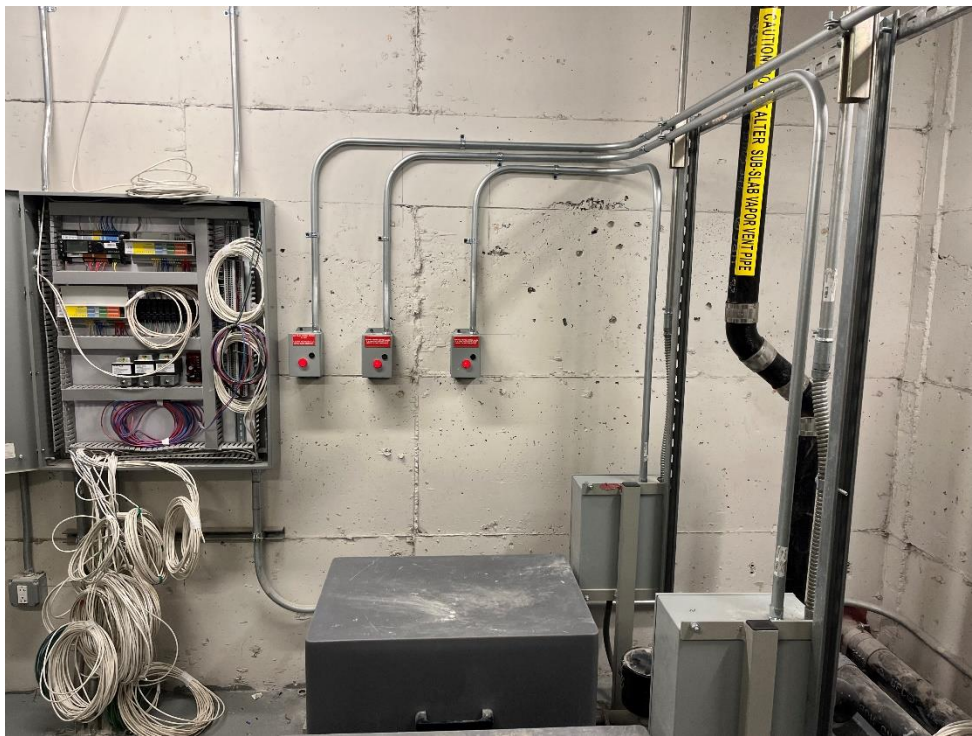
Photo 4, 01/17/2023: View of SMD system alarm panels (facing west)
