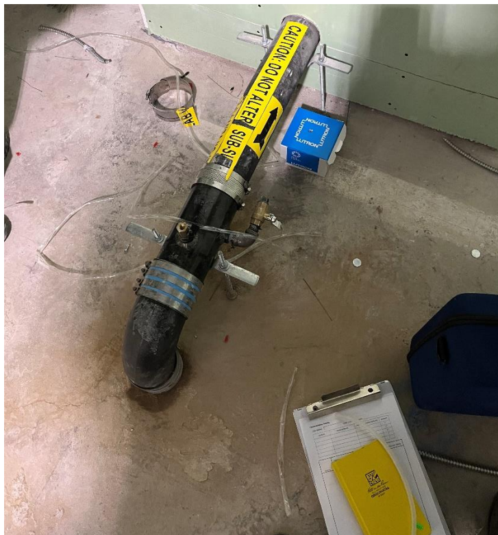
Photo 10, 01/17/2023: View of completed cellar-level riser pipe connection exiting the cellar-level slab (facing northwest)
