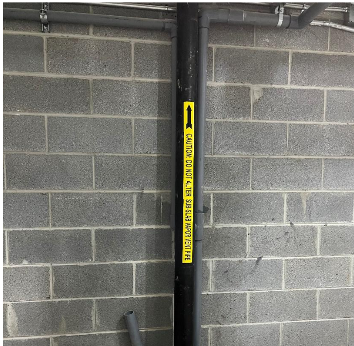
Photo 14, 01/17/2023: View of the completed riser pipe connection exiting the western first floor-level slab (facing west)
