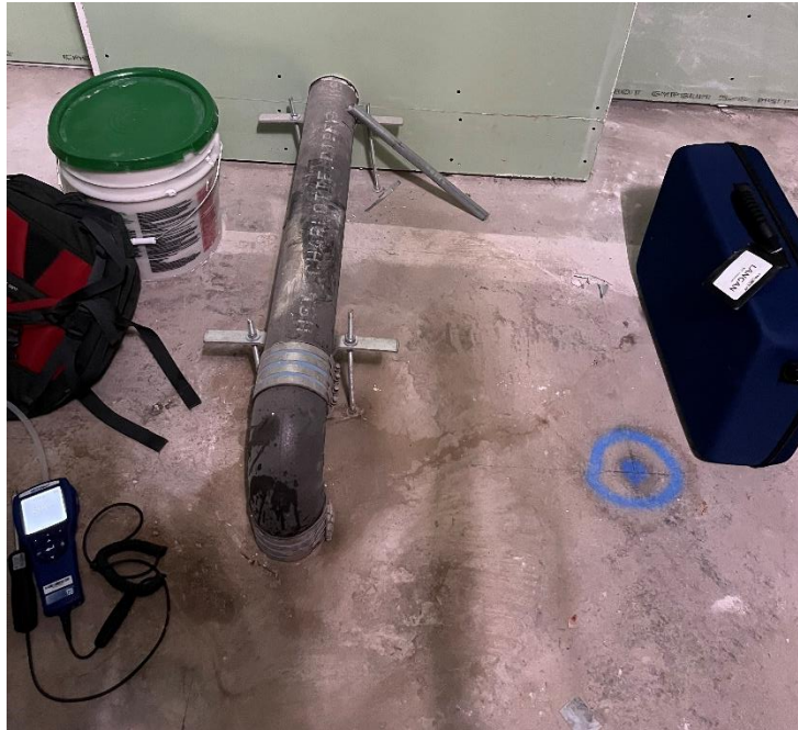
Photo 9, 01/04/2023: View of the cellar-level riser pipe connection exiting the cellar-level slab (facing north)
