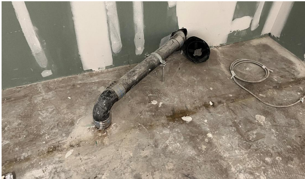
Photo 16, 01/04/2023: View of the riser pipe connection exiting the eastern first floor-level slab (facing east)
