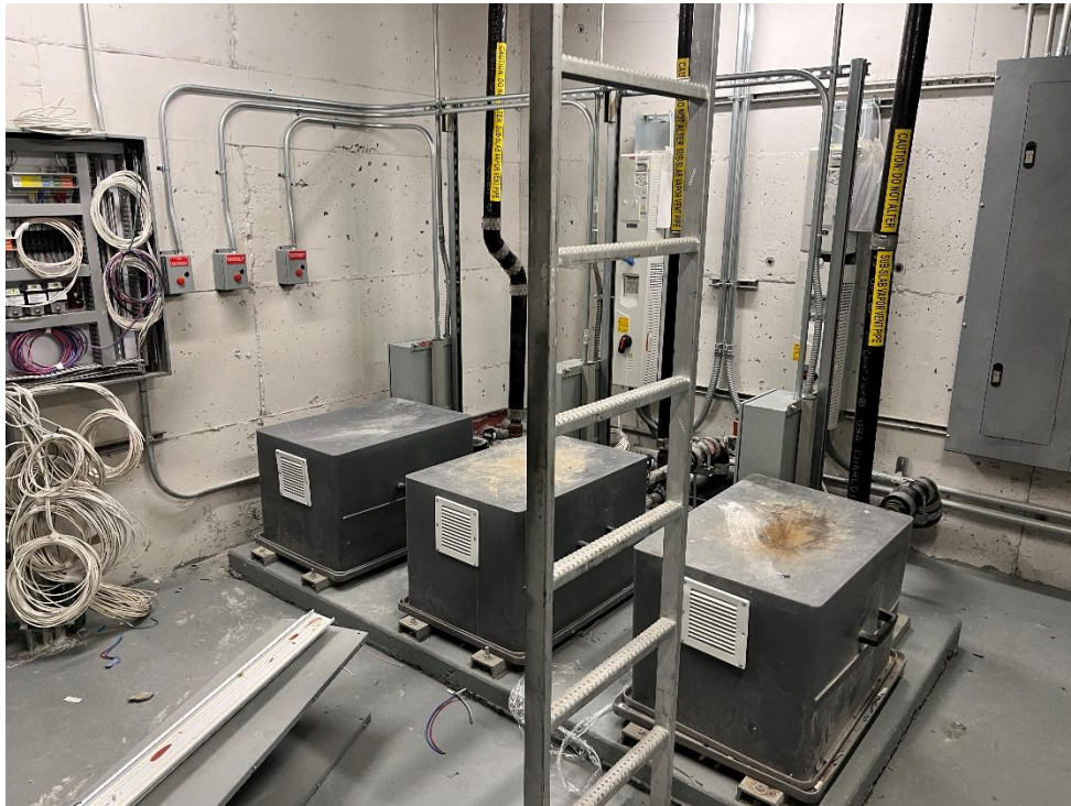
Photo 3, 01/17/2023: View of SMD blowers installed on the 2 nd level of the southern tower's mechanical bulkhead (24 th floor) (facing northwest)
