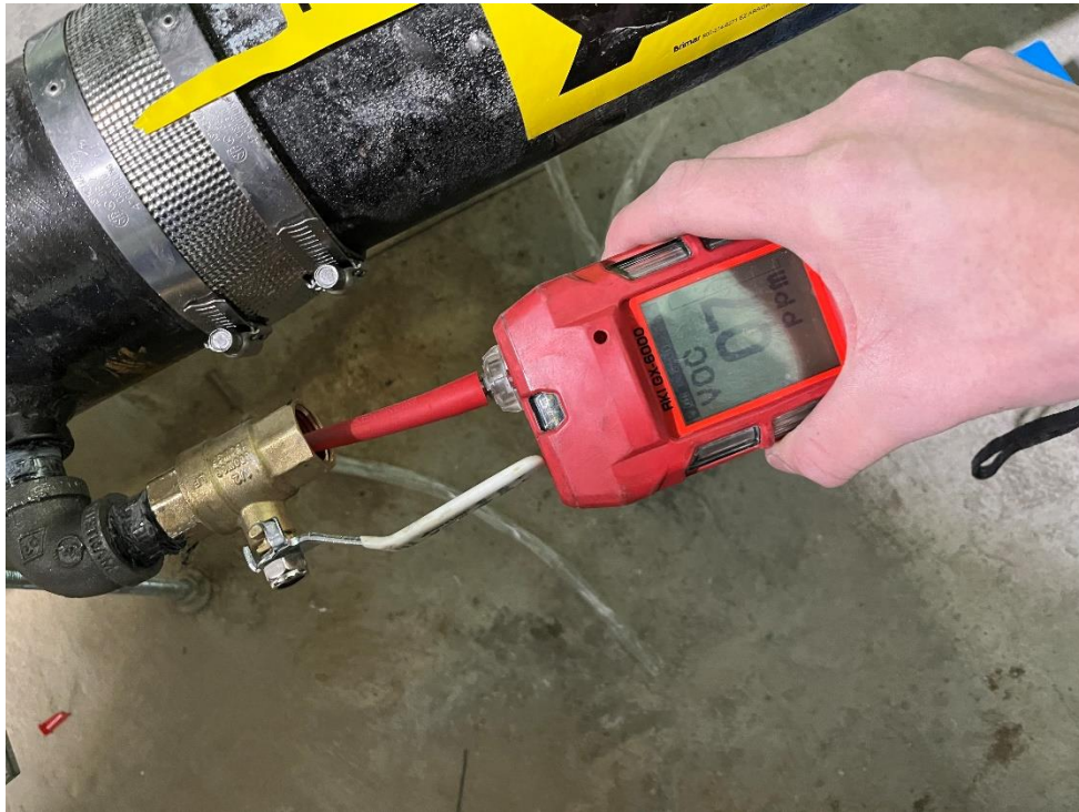
Photo 11, 01/17/2023: Langan measuring photoionization detector (PID) readings from the cellar-level riser pipe connection
