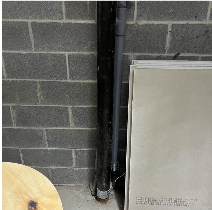
Photo 13, 01/04/2023: View of the riser pipe connection exiting the western first floor-level slab (facing west)
