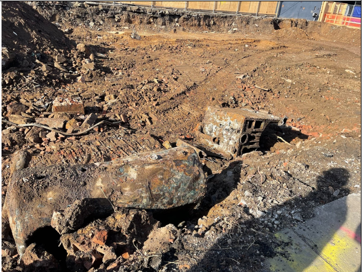
Photo 2 - View of Tank found in Zone 1 and staged for removal along Park Avenue.
