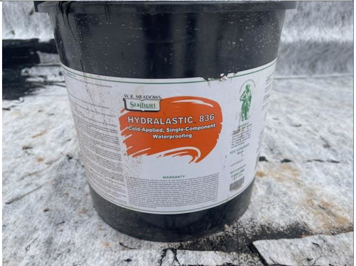
Photo 6 – View of the W.R. Meadows Sealtight Waterproofing System component Hydralastic 836.
