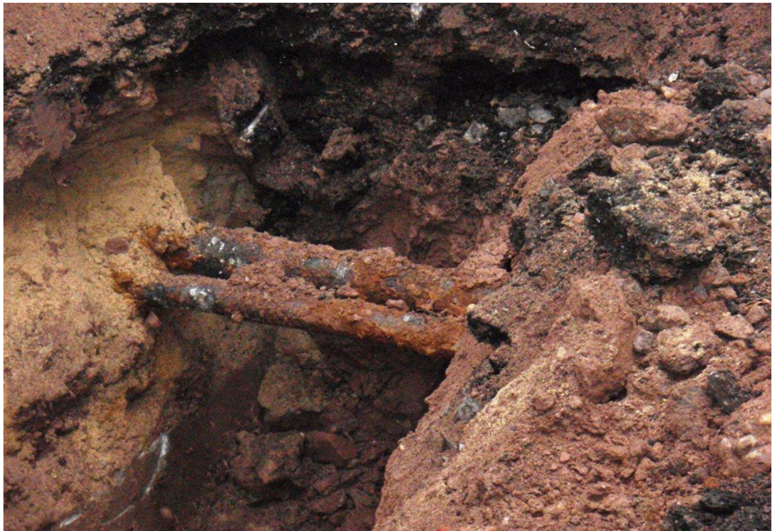
Photo 6: Piping associated with the UST was encountered at the southern end of the test pit. Facing south. 11 January 2012.
