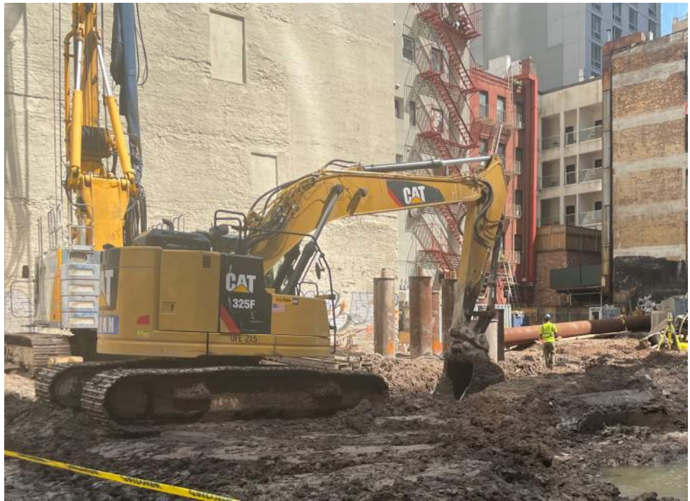
Photo 1: Urban grading soil/fill in the central part of waste characterization grid WC03 (facing southeast).
