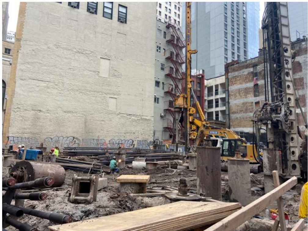
Photo 2: View of Urban drilling a rock socket at the eastern part of the site (facing east).
