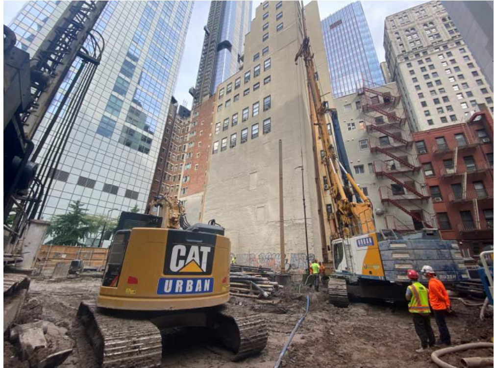
Photo 1: View of Urban grading in the central part of the site (facing northeast).
