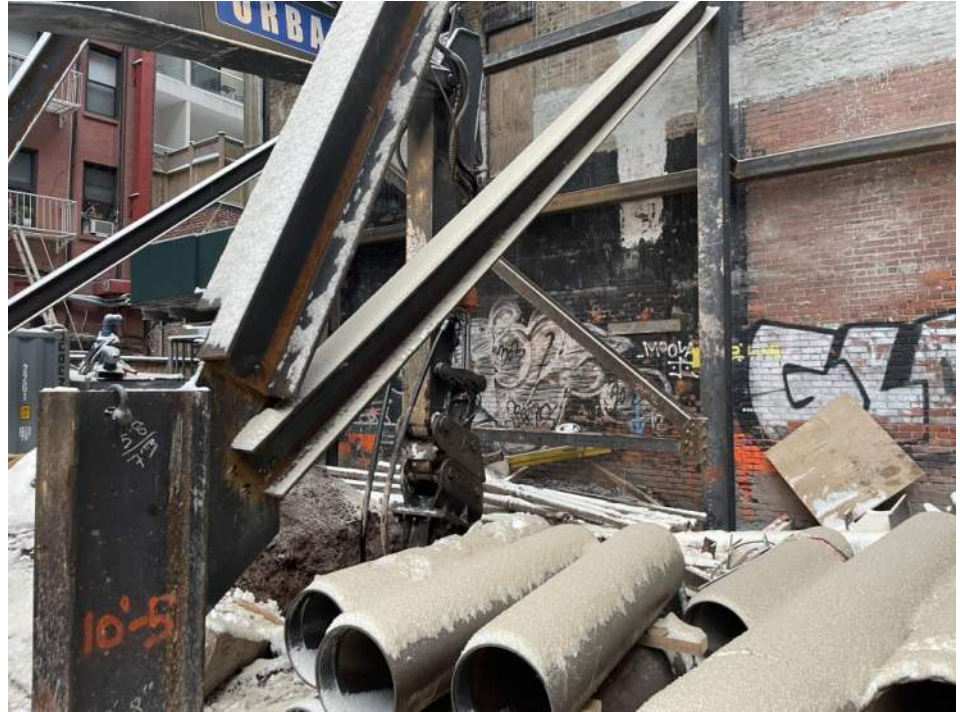
Photo 1: Urban removing concrete in the southern part of the site (facing southwest).
