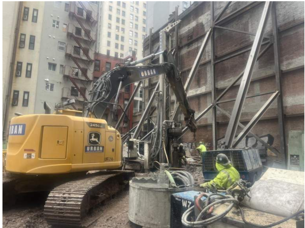
Photo 2: Urban installing a caisson casing in the southern part of WC04 (facing southeast).
