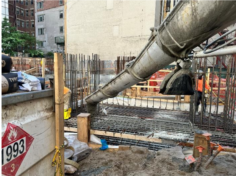
Photo 1: View of Urban pouring concrete in the southern area of the site (facing east).
