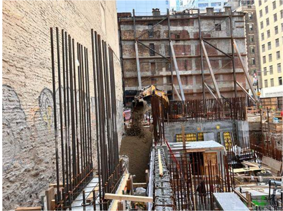
Photo 1: View of Urban backfilling clean sand in the eastern part of the site (facing east).
