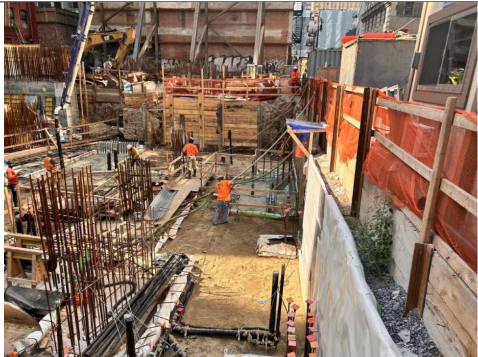
Photo 2: Urban grading soil/fill in the western part of the site (facing southeast).
