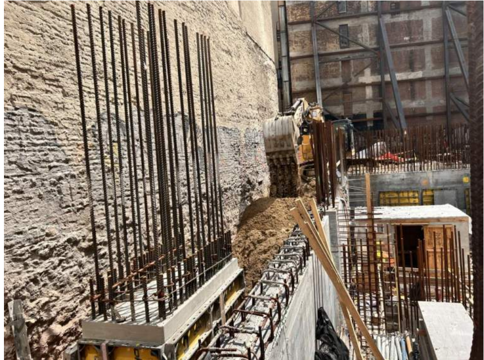
Photo 1: View of Urban backfilling clean sand in the eastern part of the site (facing north).
