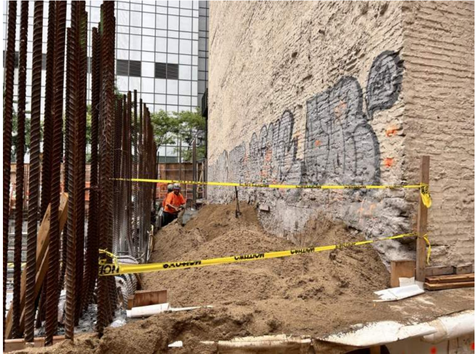
Photo 1: View of Urban backfilling in the eastern part of the site (facing north).
